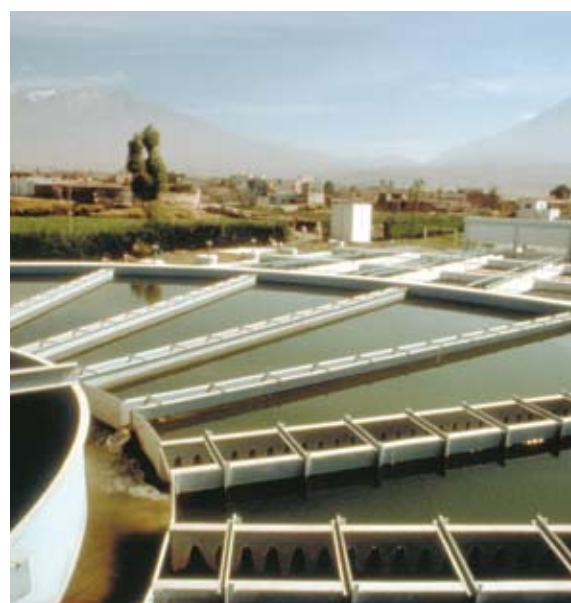
Wastewater treatment plant, Peru. Adequate treatment of wastewater prevents recirculation of pathogens in the environment.
